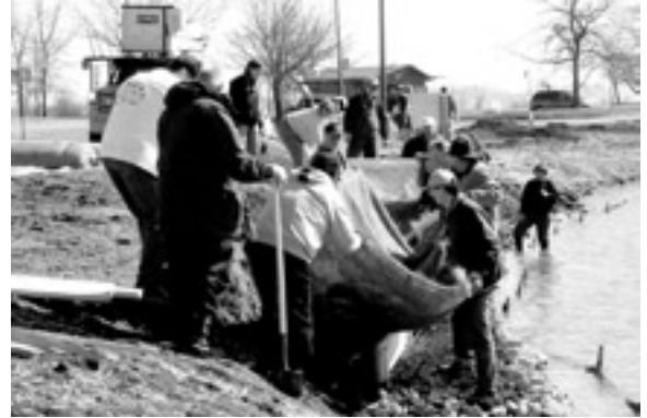
Natural Resource Conservation Service staff and volunteers install erosion control measures under a Great Lakes Basin Program -funded project along the Detroit River. (Photo courtesy Detroit-Wayne County Port Authority)
