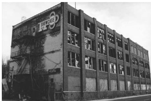
Decaying industrial building in downtown Detroit, Mich., where numerous brownfield sites await redevelopment. Photo credit: Victoria Pebbles.
