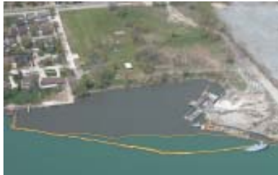
Dredging underway in the Black Lagoon. The silt curtain prevents pollutants from entering the river.
