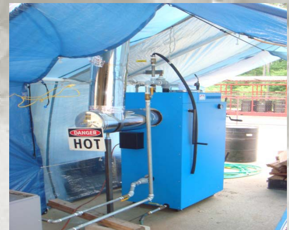
The AFB Econoburn Gasification Boiler
