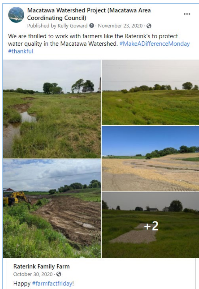
A Facebook post shared by the project team and participating producer responsible for a 635-foot two-stage channel and cattle crossing installed in an existing pasture in the Upper Macatawa subwatershed
