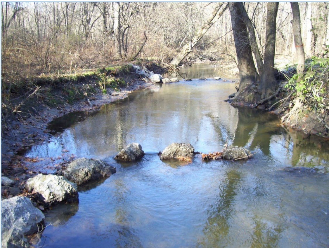
Trail Creek facing upstream at final construction of a J-hook (foreground) and cross vane (further upstream)
