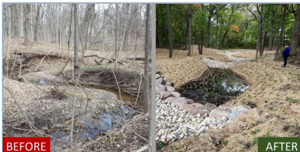
The RSC solution dissipates water energy that causes excessive erosion
