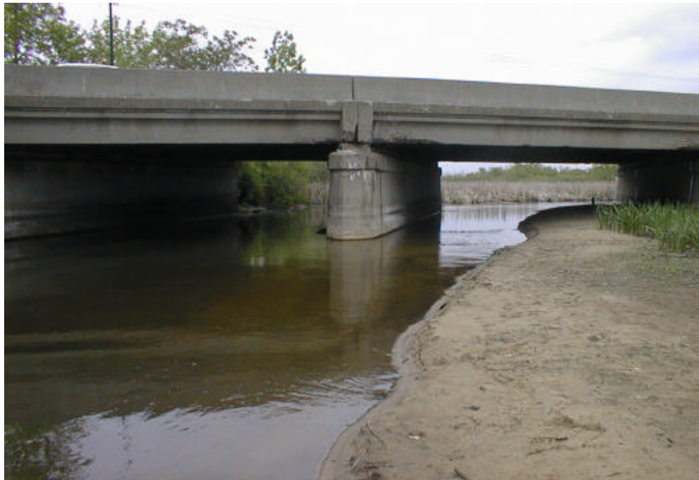
Figure 3.1.3. Large Area Of Sand Deposition Near The Bridge At Johnson Park In The City Of Muskegon.
