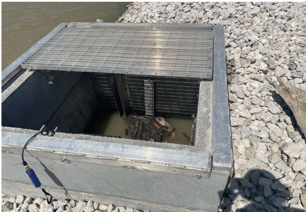
PHOTO 4: Overview of the Embayment WCS and data logger on 6/10/2022.
