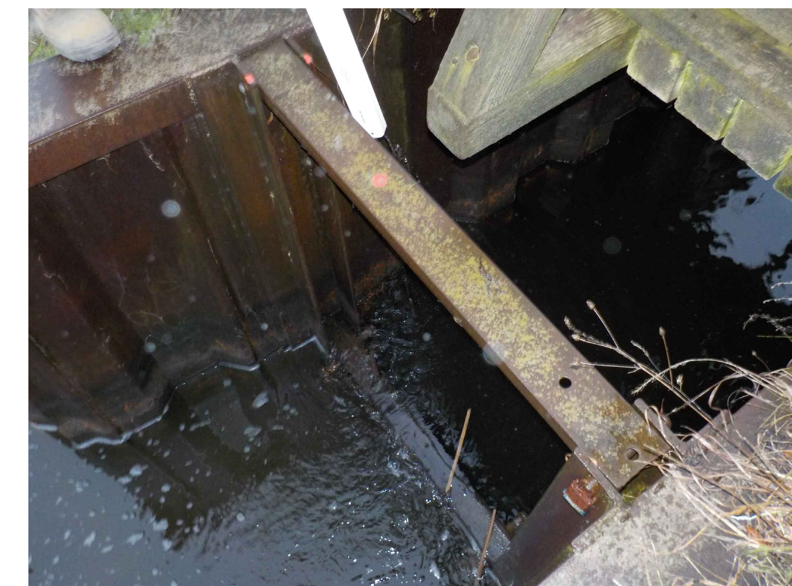
ABOVE: PHOTO OF EXISTING STOP LOG GATE TO BE REMOVED AND REPLACED.
