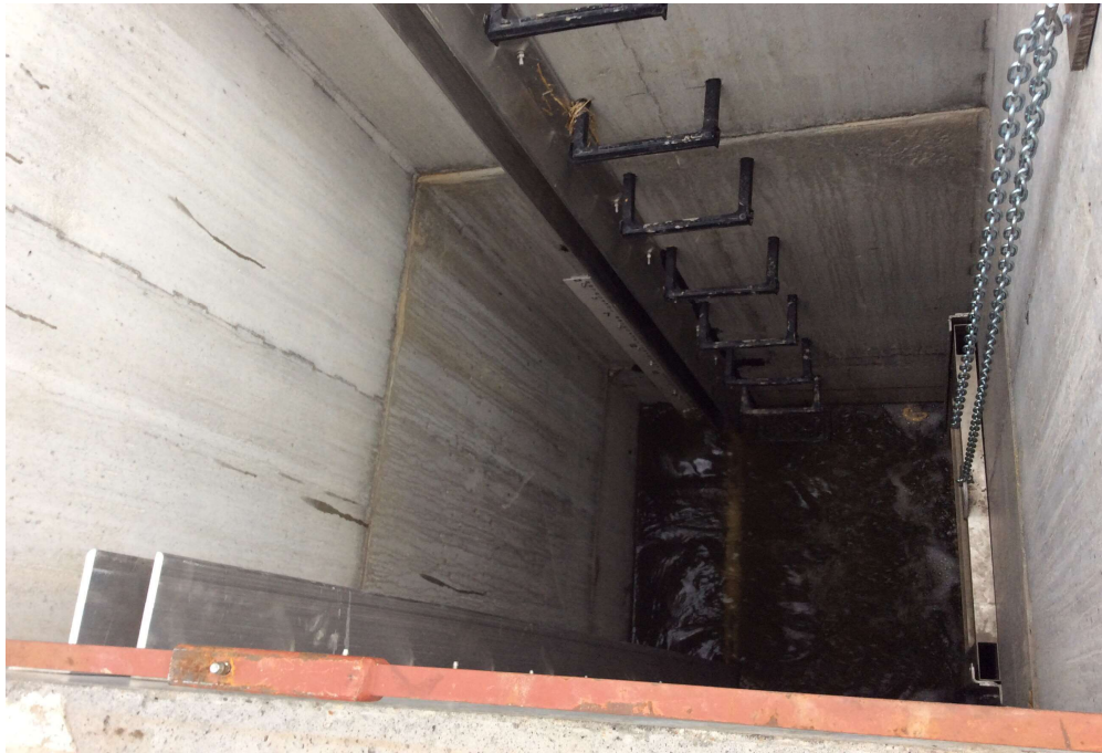
PHOTO 5: Interior of the Wetland WCS showing, from left to right, the staff gauge, stop log guides, steps, and fish grate.
